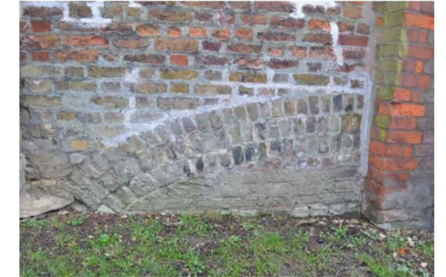
Remains of blocked culvert in west wall
